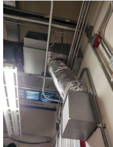
VAV BOX TAP SERVING IT ROOM
