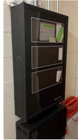
MAIN FIRE ALARM CONTROL PANEL
