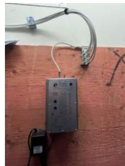
UNUSED COAXIAL CABLE SYSTEM
