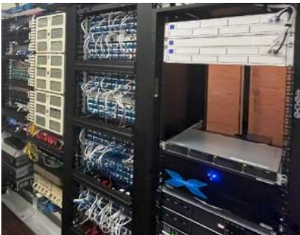
MAIN TELECOM ROOM RACKS
