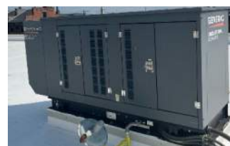
ROOF MOUNTED GENERATOR
