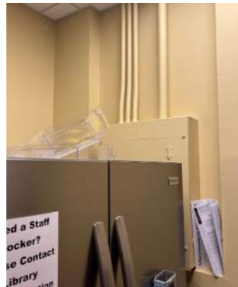
BREAKROOM PANEL WORKING CLEARANCE ISSUE
