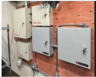
SYSTEM CONTROL PANELS AND POWER SUPPLIES
