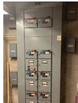
TYPICAL MOTOR CONTROL CENTER
