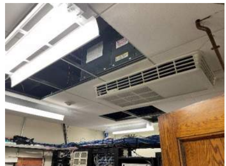
FAILED COMPUTER ROOM UNIT
